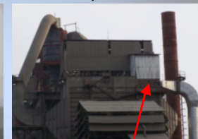
Precip Filter installed in last ESP field (field emptied of its internals) ESP now housing 2 Fields Plus "Precip Filter" (Clean Environment)
