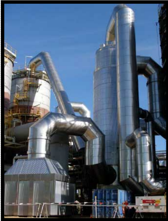
Sulphuric Acid 100,000 TPA
